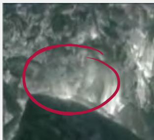
Gas leak on land fill surface
