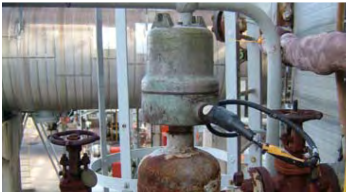
Level float switch
