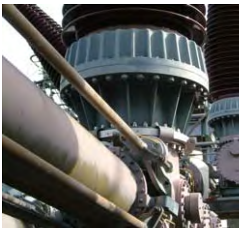
Figure 1. Typical SF 6 Filled Substation Equipment
