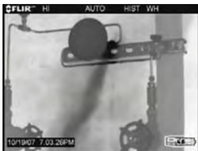
A leaking pressure gauge
