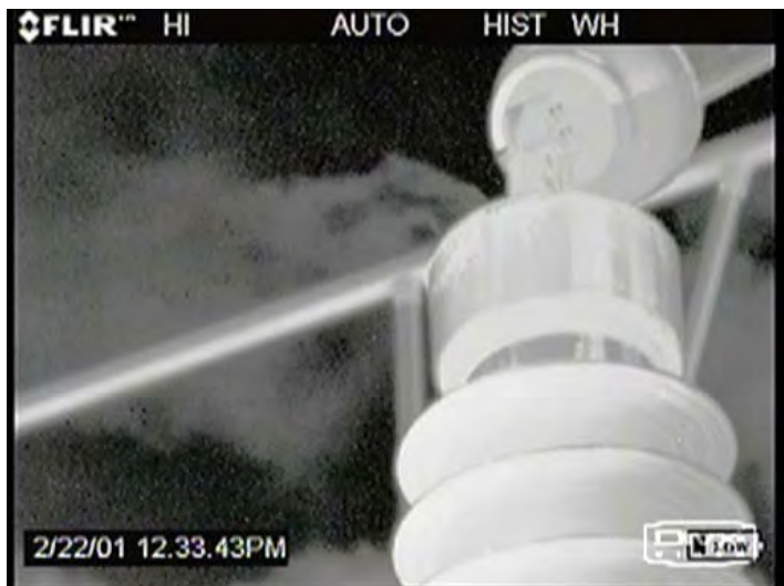
SF 6 leak from a high voltage insulator
