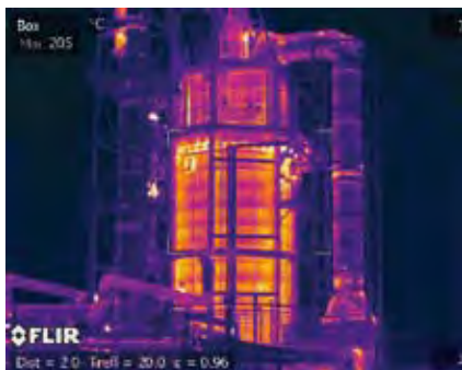
Infrared image of a process furnace
